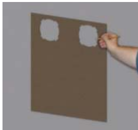
Mark the holes for the air ducts with a cardboard master plate.
