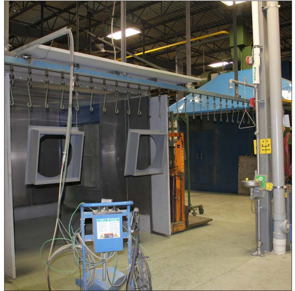
Power Paint Line, Brockville plant. (2009)
